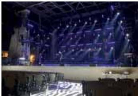
IPS AVL Power Control from LynTec for the FirstBank Amphitheater set in a former Tennessee Rock Quarry.
